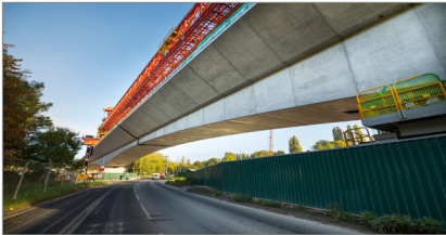
Completed A412 road crossing between P55 and P54 with a grout connection at the Colne Valley Site, October 2022
